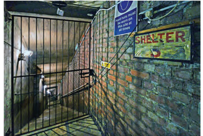
At the top of the south side wartime access stairs, where the reinforced concrete ceiling shows how close to the surface, and thus more vulnerable, it is
